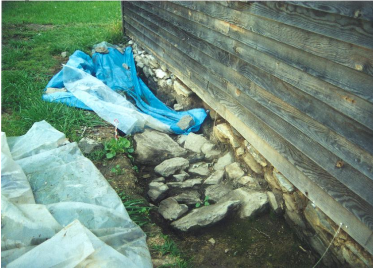
Excavation, along east wall of original house, showing porch stoop under W 105 (October 1999) - IACPH71.htm
