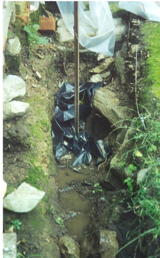
Excavation, along west wall of original house, showing stone foundation running parallel to original one (October 1999). - IACPH70.htm
